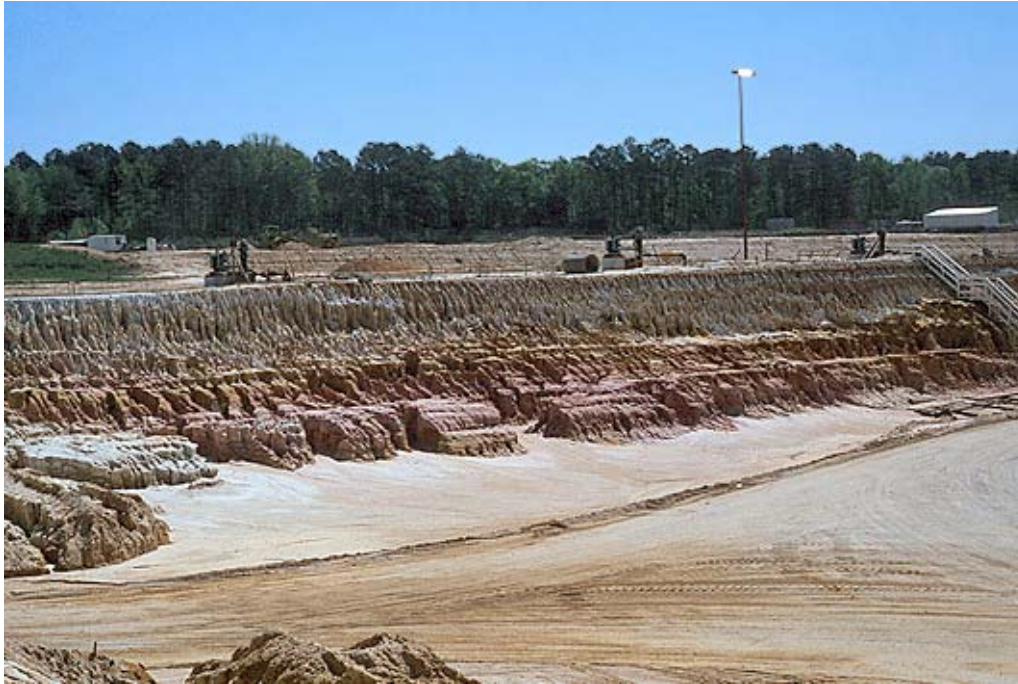
Figure 3.2.2 Close up of bench cuts in silt material along the edge of the excavation. Three dewatering wells are seen along the perimeter of the excavation.
