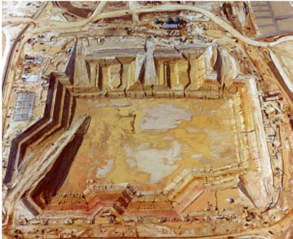
Figure 3.2.1 The 41-acre 100-foot deep excavation at River Bend station created for construction of the nuclear power plant and other structures had bench cuts at the edge of excavation. The access ramp is seen on the bottom left of the photograph.
