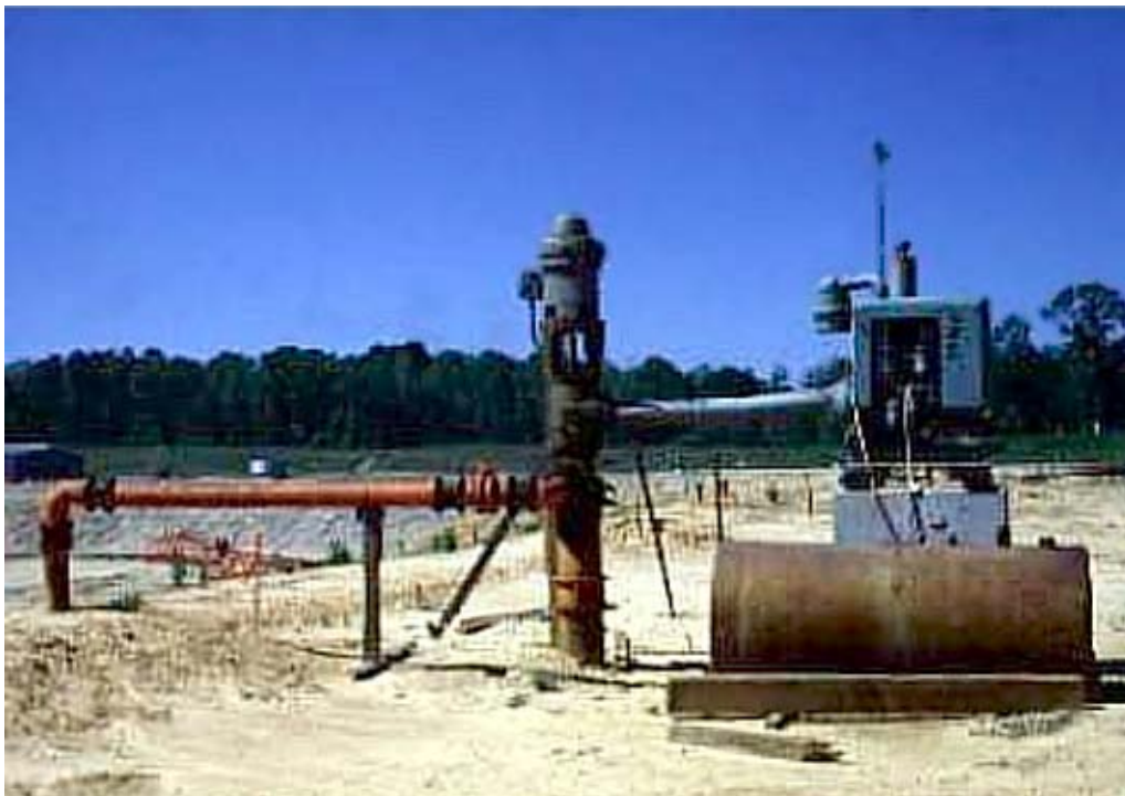
Figure 3.2.3 One of the 44 dewatering wells surrounding the excavation at River Bend station.
